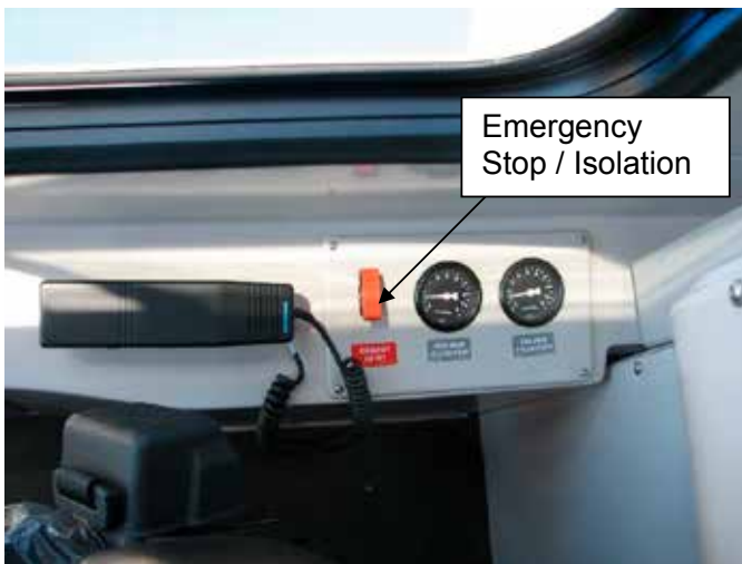
Figure 2-12 Location of Emergency Stop / Isolation Switch
